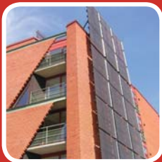
Solar tubes on apartment block generating hot water
