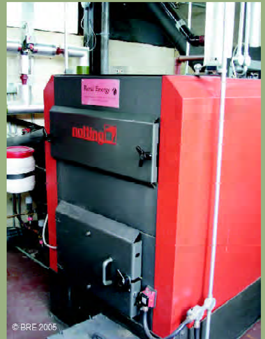
A biomass boiler suitable for serving a group of dwellings
