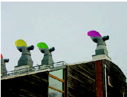
Ventilation cowls draw out hot air providing natural ventilation by the 'stack' effect - BedZed
