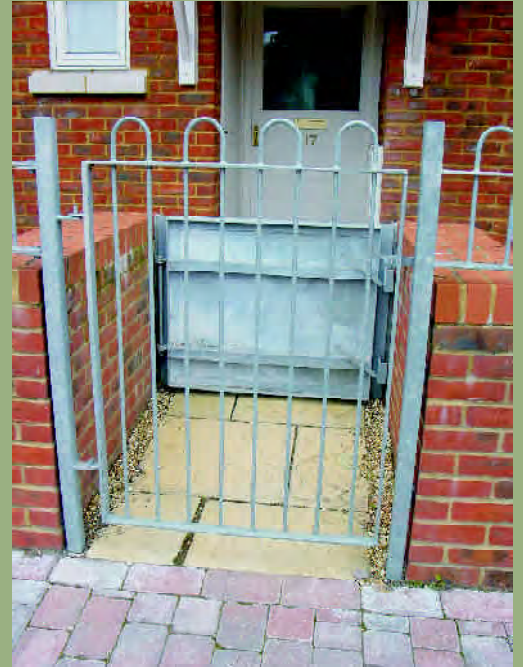
Flood gates fitted to boundary walls of 225mm thickness to provide resistance to potential flooding of individual terraces - Hythe
