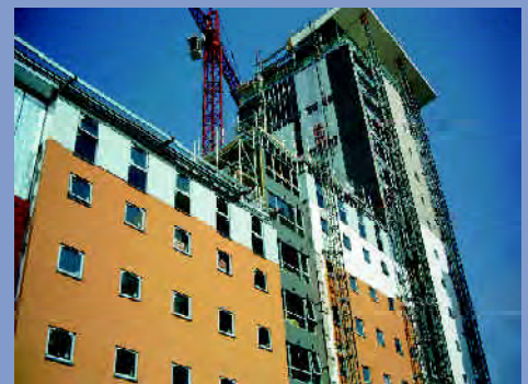
Off site pre-fabrication of units can reduce costs and construction time on site, however care must be taken that cladding materials are appropriate for the context and well detailed - Mercury Point, Southampton
