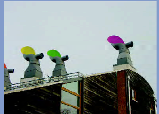
Ventilation cowls are designed as an integral feature of this sustainable development - BedZed
